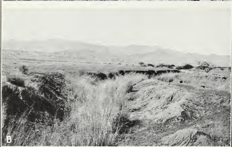
A.—Flood control fence constructed with iron posts to reduce velocity of flow, induce silting, and prevent bank cutting in a large drainage (Arizona) B.—The establishment of grass in a gully tended to check further cutting (Arizona)
